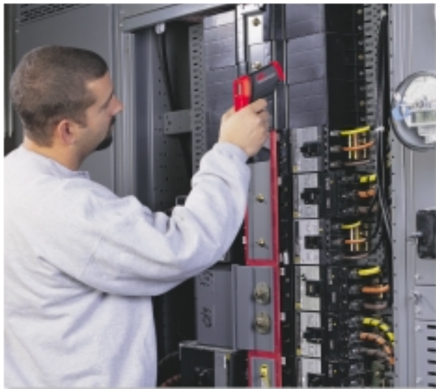
Check for hot spots in electrical panels and circuit breakers, generators and gearboxes.
