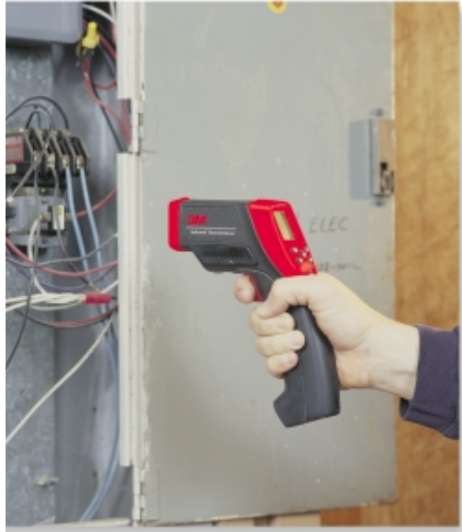
Store temperature measurements for more precise monitoring.
